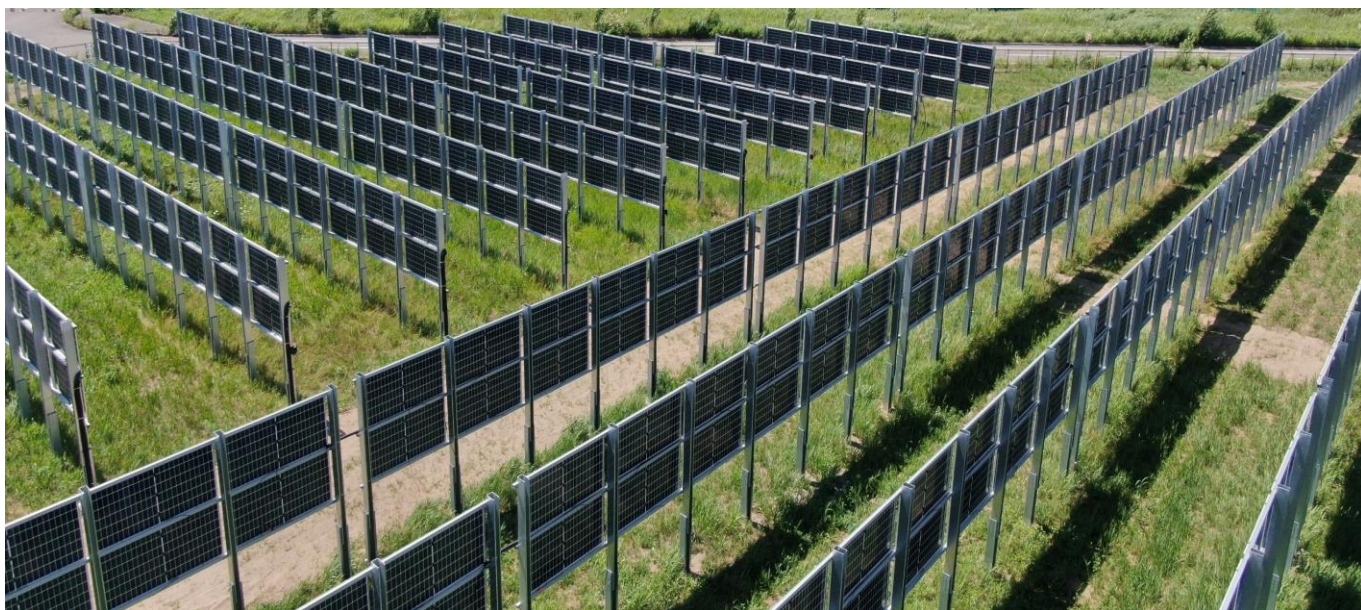
Exterior view of vertical solar power generation facility
