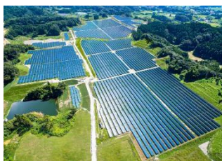
ReENE Chonan Solar Power Plant (Chonan, Chiba)
