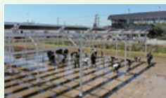
ReENE Solar Farm Higashimatsuyama
