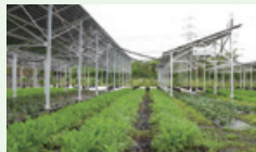
ReENE Solar Farm Higashimatsuyama
